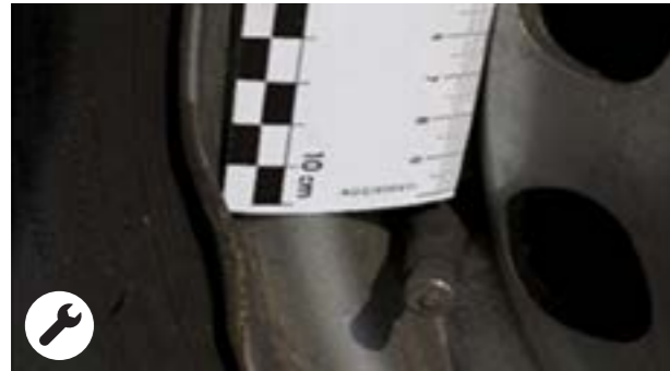
On steel rim: Attachment edge slightly deformed
