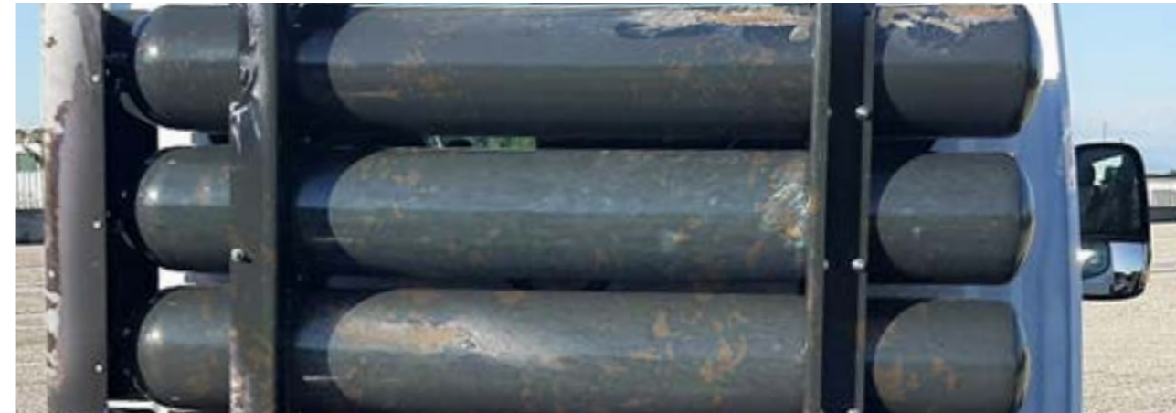
Evidence of repairs to the CNG cylinder → charge for replacement for CNG cylinder.
