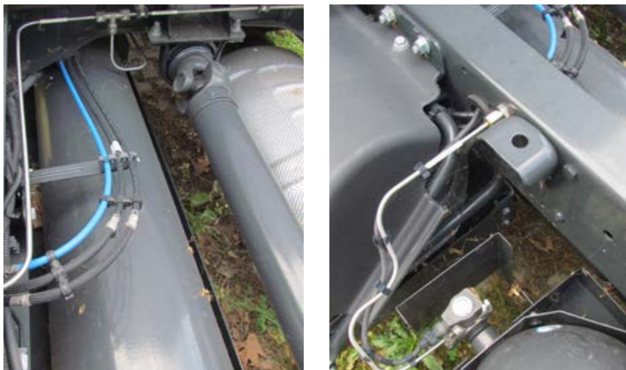
Check integrity of the gasoline fuel lines (no losses, no evidence of deep scratch). Fuel lines must be returned in proper conditions as illustrated in picture.
