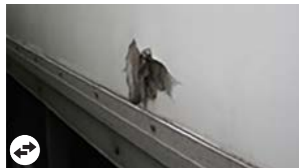
Wood side panels: Damaged wood support \geq 20 cm
