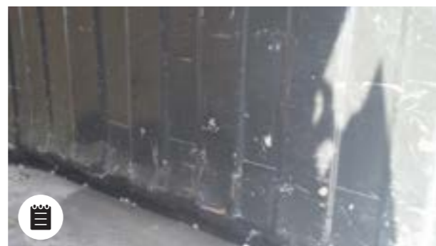
Internal deformations: Slight deformation without perforations or cuts, repair time ≤ 3 h
