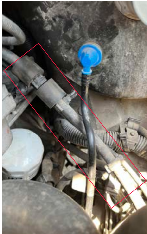
Cuts/scratches/gouges/abrasions • charge for replacement of medium pressure pipe.
