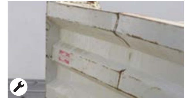
Deformations in the body closures with a repair time > 1 h within economic repair
