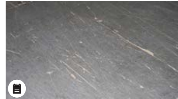
Flooring: Slight deformation, superficial wear
