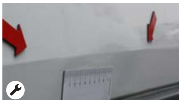
Defect: Deformed panel following repair
