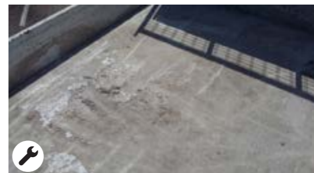
Trace of concrete or chemical product covering \geq 1/4 of the surface of the bed
