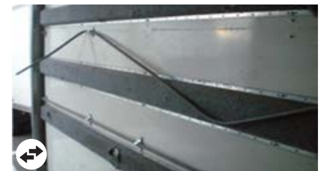
Upholstery and rods: Rods, fastenings, upholstery missing or deformed beyond economic repair
