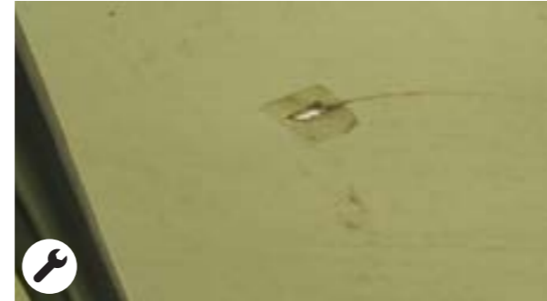
Roof space: Perforated or torn within economic repair
