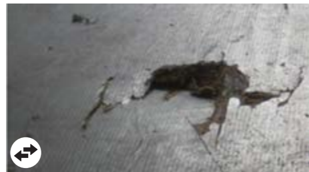
Flooring: Deformations or perforations within economic repair
