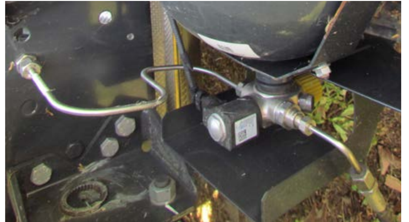
Rust, dents, breakages and/or gouges • charge for replacement of rigid lines.
