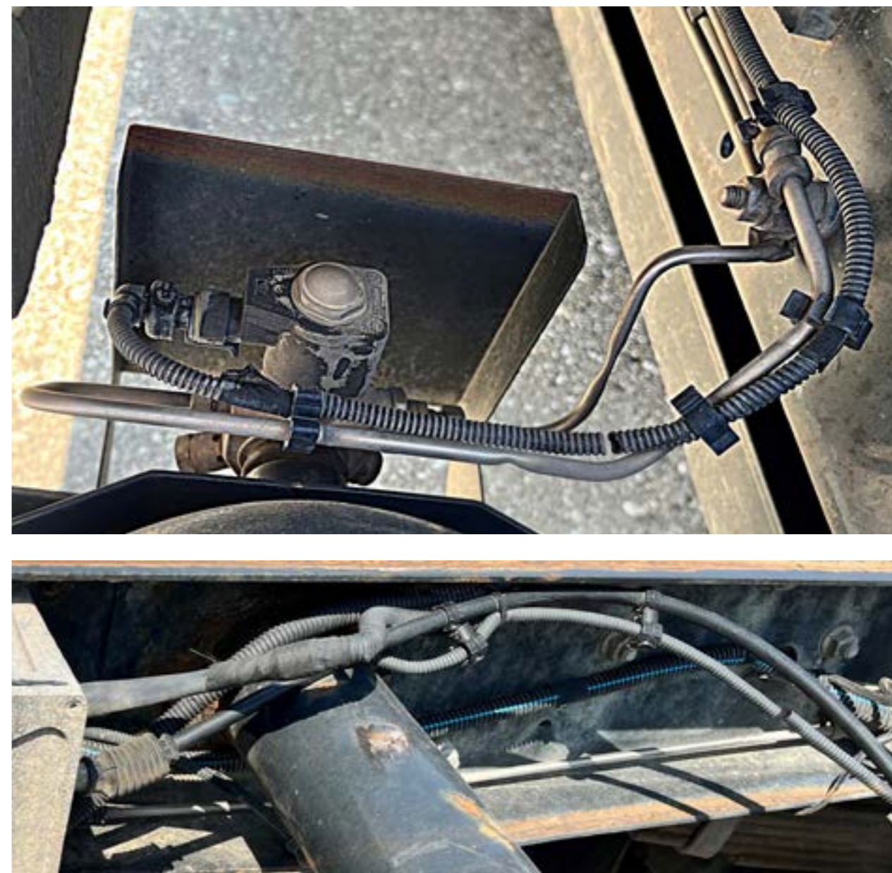
Losses or evidences of deep scratches • charge for replacement of fuel lines.
