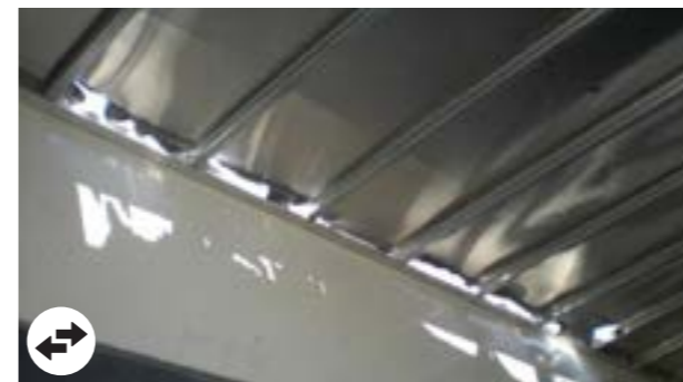
Roof space: Frame damaged, leather not within economic repair
